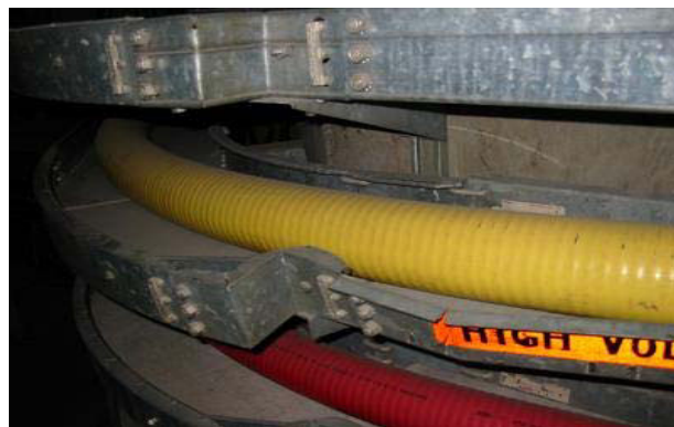
Fig. 1. A typical installation of a power cable in a tunnel at the University of Washington.
